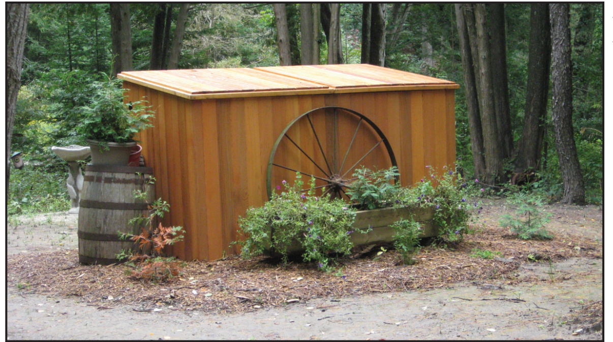
SEWAGE TREATMENT IN DISGUISE. This attractive cedar shed houses the Waterloo Biofilter System's trickle filter for treating sewage effluent before releasing it back into the ground. The above-ground system is perfect for cottages surrounded by rock or for properties with limited space. (Submitted photo)
