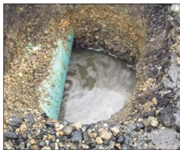
Wastewater stands in the failed pressure distribution disposal field.
