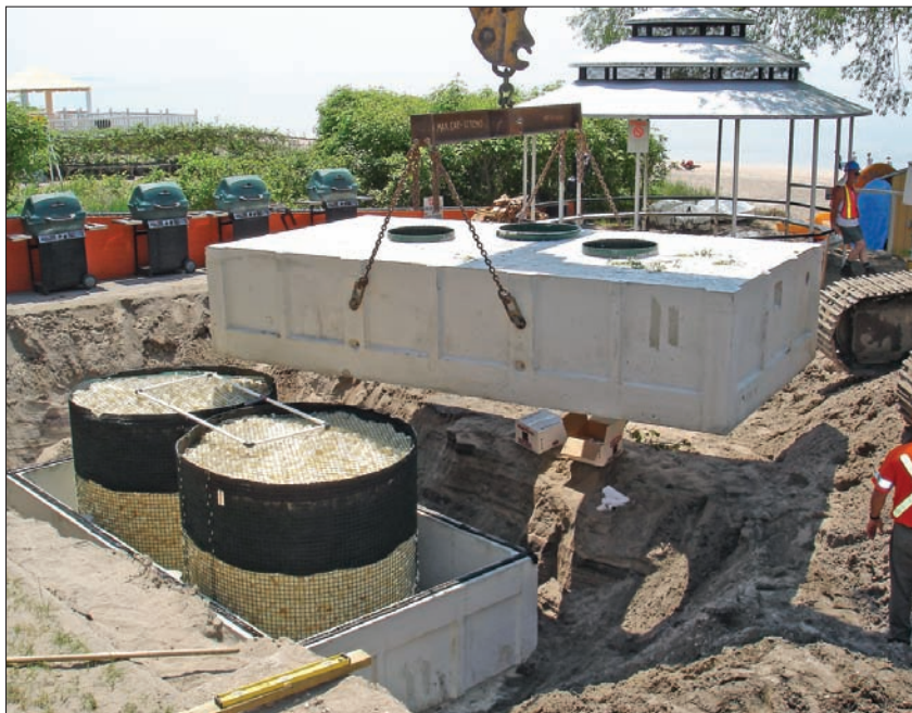
A crane operator places the top of the biofilter container tank over the foam media and distribution system.
