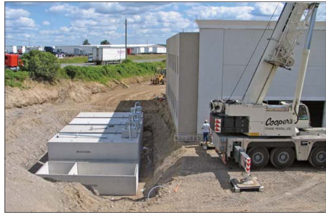
A crew places the last of five 13,200-gallon water reservoir tanks for fire-fighting in the north end of the property.
