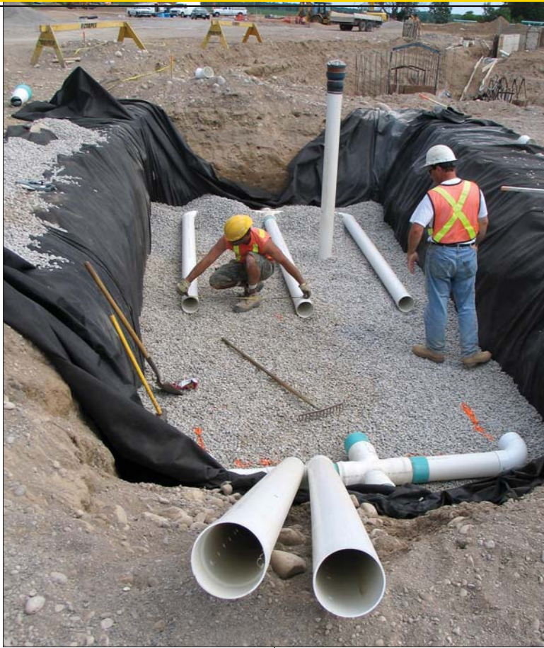
John Van Neiuwenhuizen (left) and Dave Mc Cready from D.W. Cooper Contracting install a rainwater infiltration gallery.
