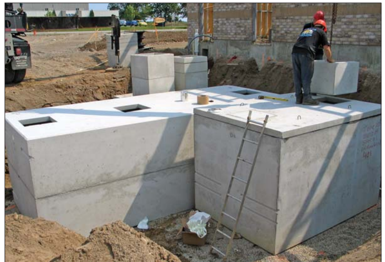
The crew from Unit Precast places (background to foreground) the kitchen holding tank, grease interceptor, and one pump tank.
